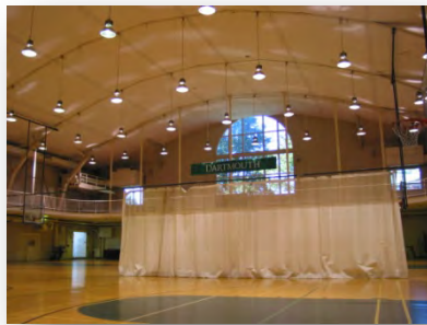
Original West Gym lighting system
